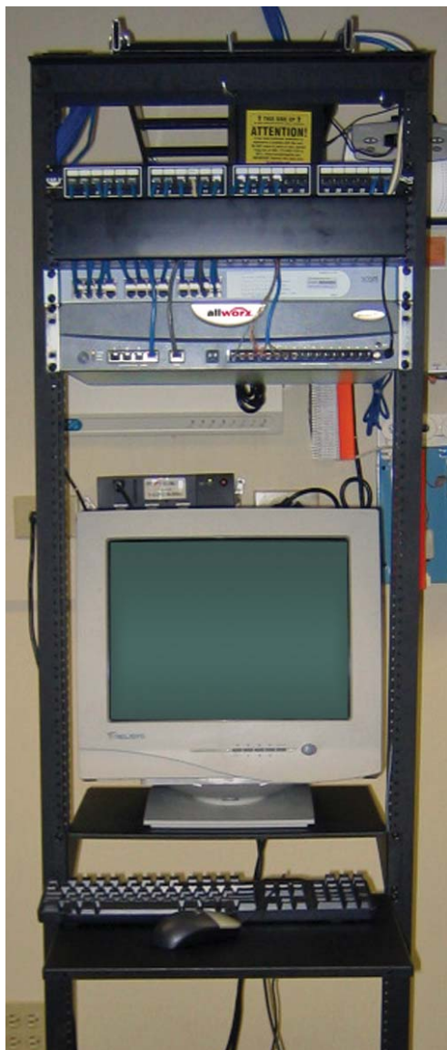
The Allworx 10x is the hub of Abram Law Group's technical infrastructure, providing protection and networking capabilities.
