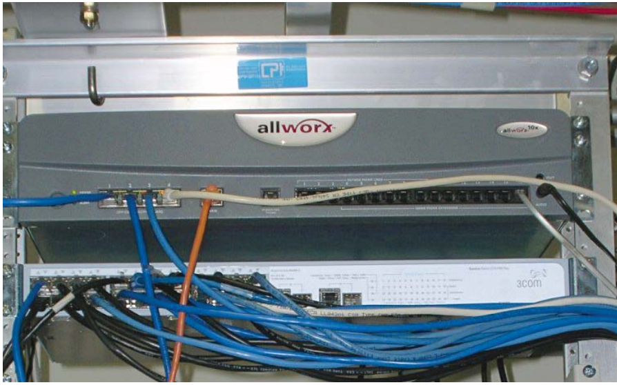
Allworx is the hub of MZI HealthCare communication system. The Allworx 10x is shown above connecting the PBX phone system, Local Area Network and Internet. The Power Fail analog phone is above to the right.
