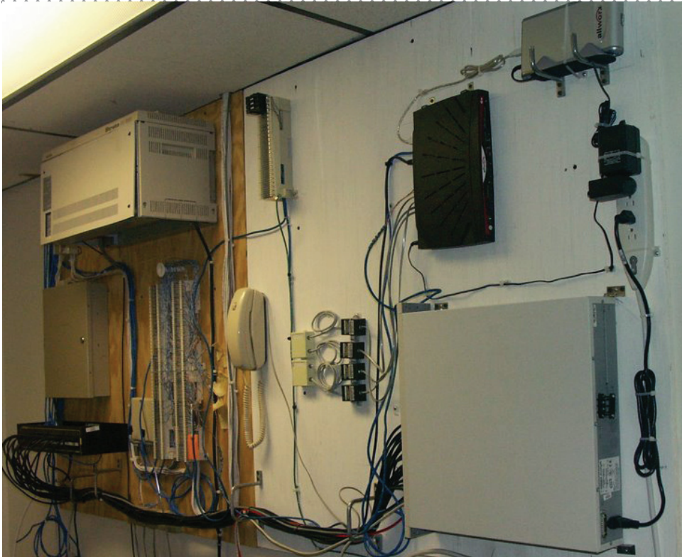
The Allworx 6x is shown above connecting to a T-1 Line, router, server, the Allworx USB hard drive, and the Internet to create the hub for United Security's communication system.
